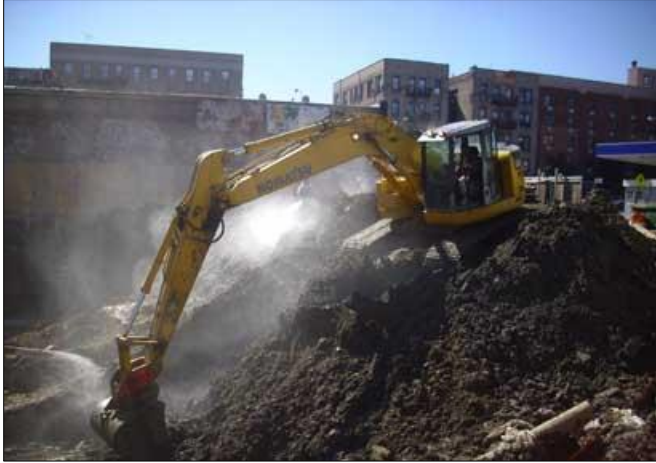
A brownfield site in Bronx. Photo courtesy of the Mayor's Office of Environmental Remediation.
